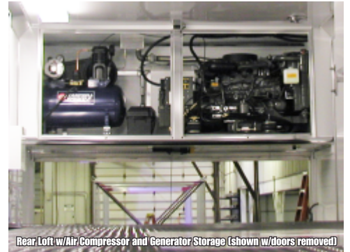
Rear Loft w/Air Compressor and Generator Storage (shown w/doors removed)
